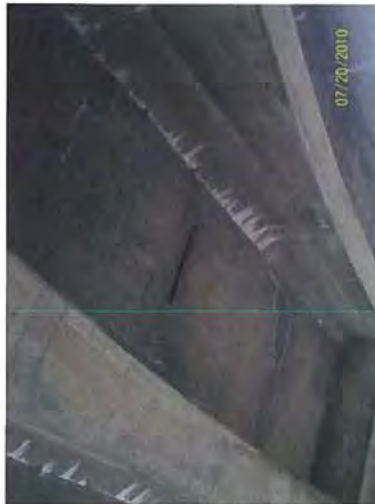
Concrete spall with exposed rusting reinforcing steel noted in bay 2, span 3.
