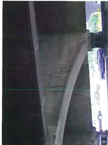
Exposed rusting reinforcing steel noted in beam # 2, span 1.
