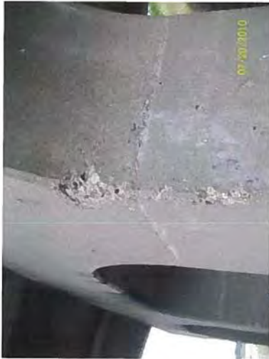
Traffic impact noted in pier # 2, column 1
