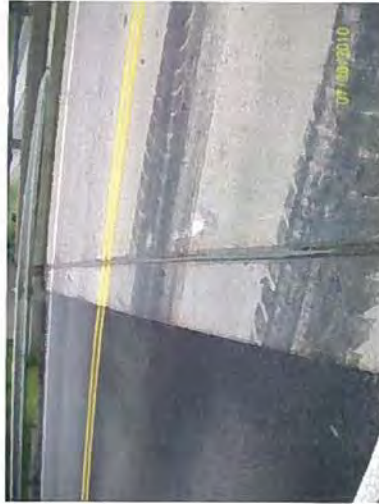
Compression joint noted at the forward transition.
