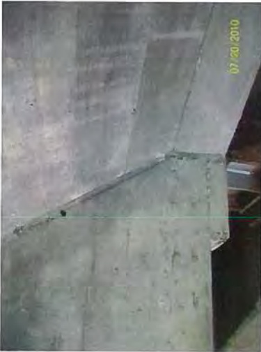
Open cracking noted at beam end # 3 at forward abutment.
