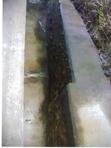
Roadway dirt and debris noted in rear abutment seat.
