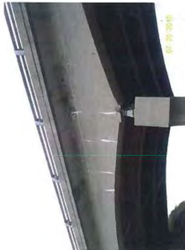
Vertical flexure cracking with efflorescence noted in exterior beam # 4.
