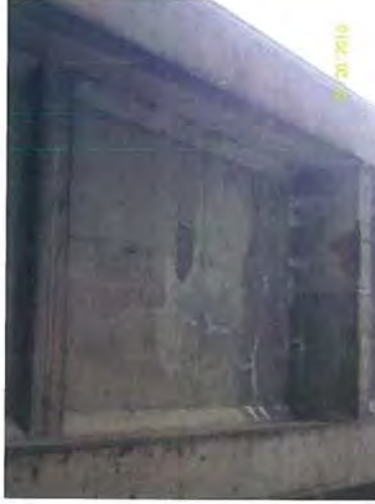
Concrete spall noted in deck soffit, span 2, bay 3.
