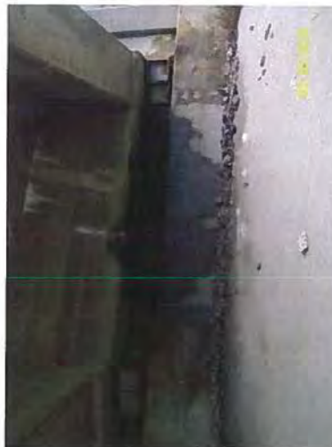
Seepage noted in abutment seat at forward abutment, right side.
