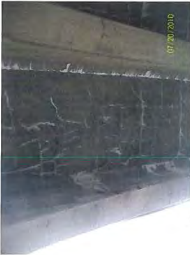
Diagonal, longitudinal, and transverse cracking with efflorescence noted in bay 3, span 2.
