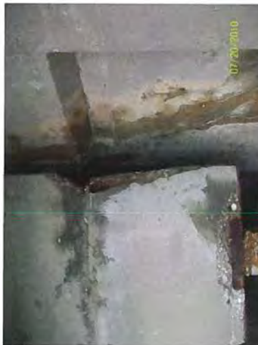
Concrete spall and exposed rusting reinforcing steel noted in beam end # 4 at forward abutment.
