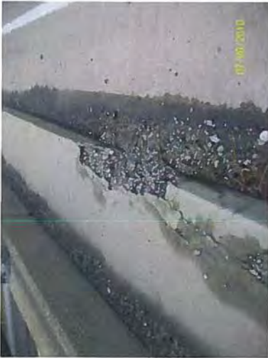
Concrete spall and exposed rusting reinforcing steel noted in concrete curb element, right side.
