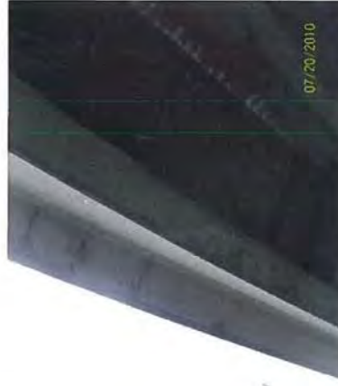
Traffic scrape noted in span 3, beam 1.
