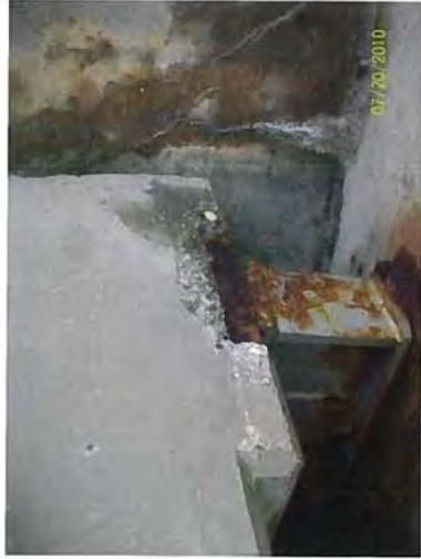
Concrete spall found typical throughout beams at sole plate.
