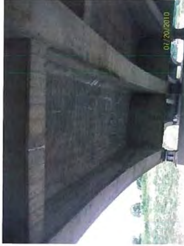
Longitudinal cracking with efflorescence noted in deck soffit, span 4, bay 3.
