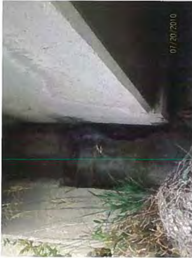
Concrete spall and exposed rusting reinforcing steel noted in back wall, right side.
